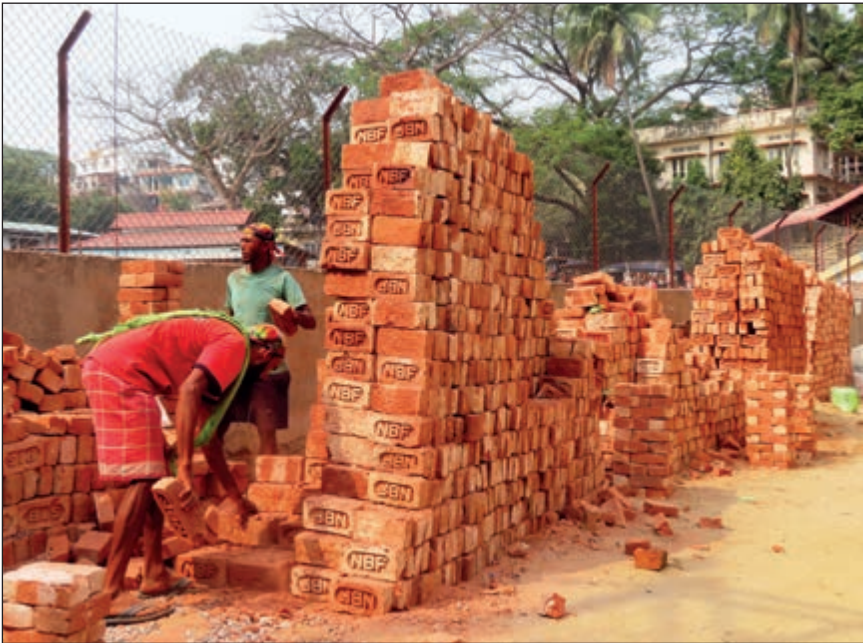
Abbildung 3: Baustelle in Hyderabad, Indien; Foto: Autor 2017. Figure 3: Construction site in Hyderabad, India; photo: author 2017.
